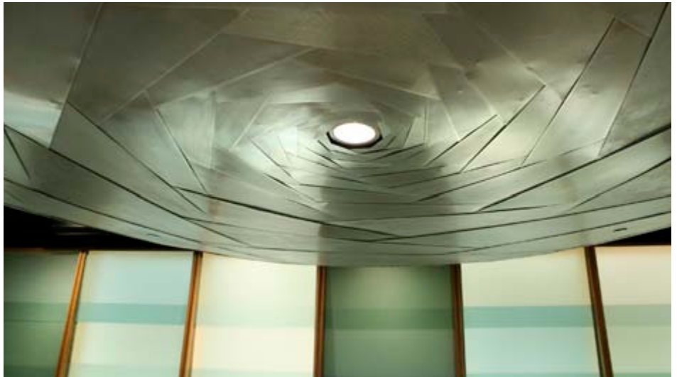
Layered aluminum laid in a circular pattern form an aperture for the lights.
